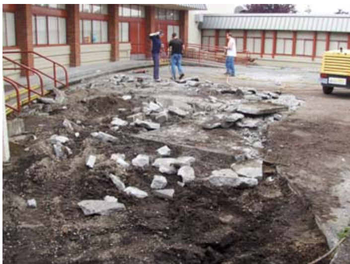
TSFT members, with construction professionals, pulling up and recycling concrete to prepare the courtyard for construction of the Rain Garden - August 2007
